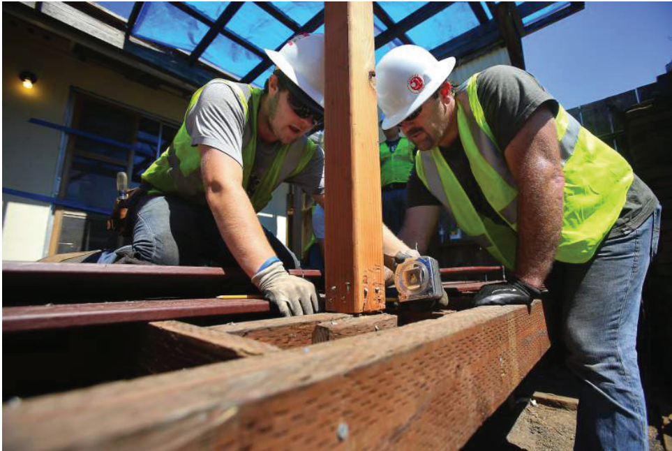
North Bay Construction Corps "Pathway to Paycheck" Boot Camp participant Pat Ojeda, left, takes measurements with the help of Larry Richmond, Jr., who is volunteering as a mentor and trainer, as they rebuild a patio at a home for a Habitat for Humanity "Elder Care Project" in Santa Rosa on Wednesday, June 21, 2017. (Christopher Chung/ The Press Democrat)
